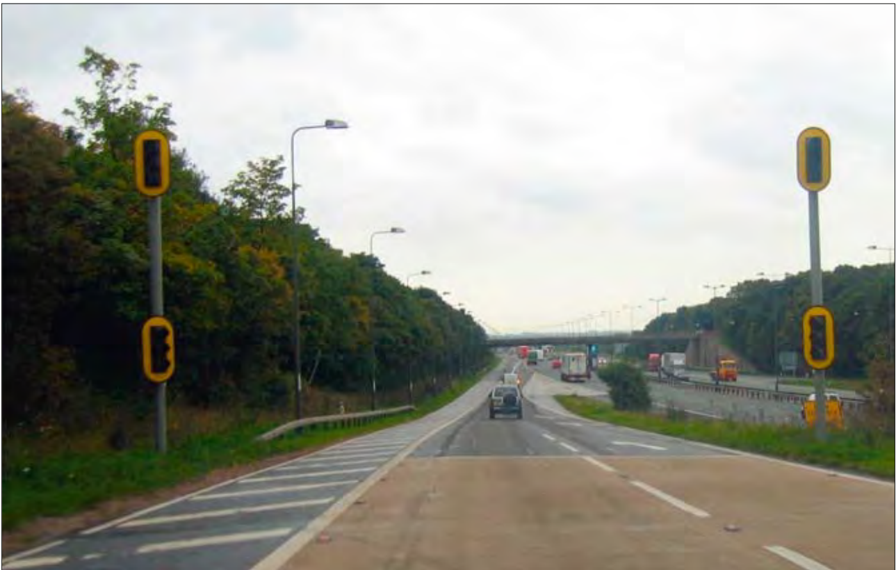
Figure 6.1 Ramp metering signals
